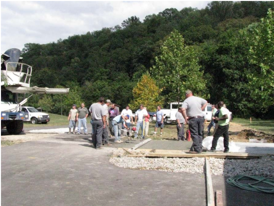
STUDENTS FINISH STRIKING OFF THE LAST OF THE PERVIOUS CONCRETE PAD USED FOR THEIR HANDS ON PLACEMENT
